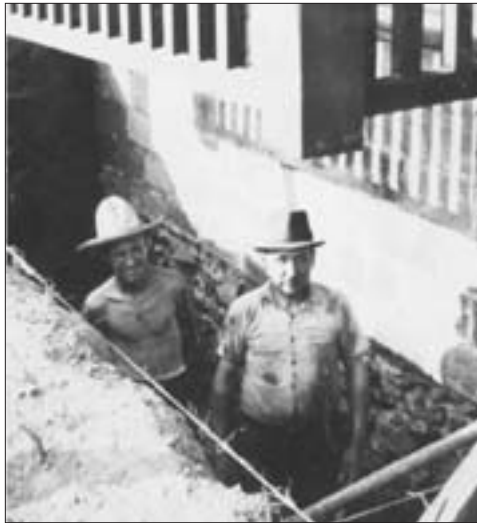
John Alzo, Sr. (right) was a "jack-of-all-trades". He is seen here with his son, John, Jr. when they were building a coal bin for their house.
